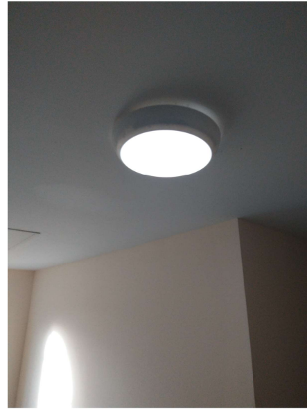
Lighting (Standard and Emergency Lights)
